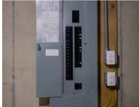
200 amp electrical service
