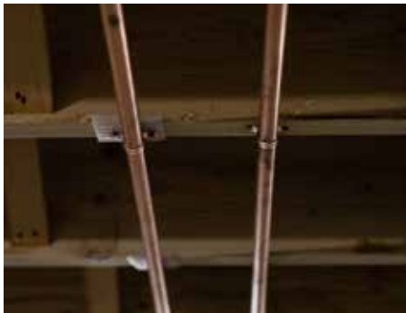
Copper plumbing & water lines with 3/4" supply lines, two (2) exterior hose bibbs
