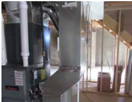
Cold air return system
