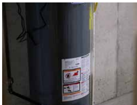
50 Gallon high efficiency hot water tank
