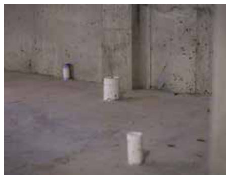
Rough-in plumbing for a future bathroom in basement
