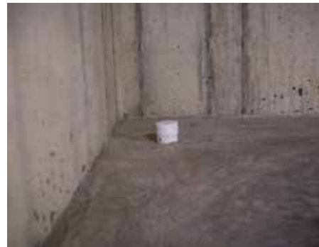
Interior and exterior french drains
