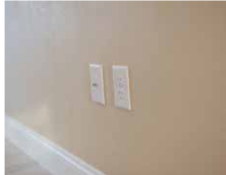
Five (5) phone & (5) cable outlets
